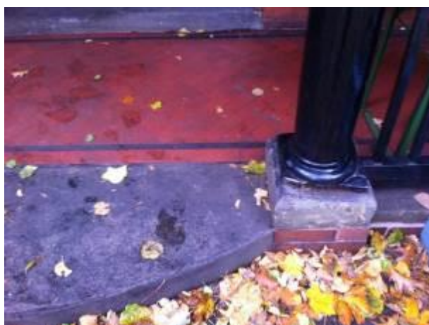
Damage to base of timber column by main entrance
